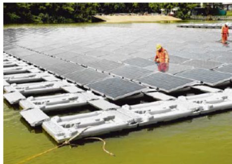
The floating solar panel test bed at Tengeh Reservoir is the world's largest. PUB is looking at adding solar systems to Bedok and Lower Seletar reservoirs to power its energy-intensive water treatment processes in a greener way. ST FILE PHOTO
